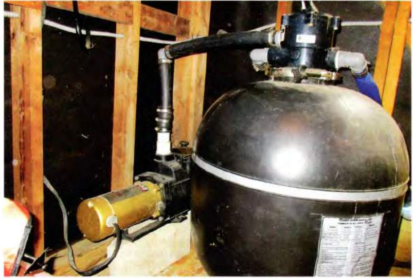
A quick visual inspection of all the equipment located above ground (i.e. pump, filter, heater, and hoses) should be performed as part of the preliminary investigation.
